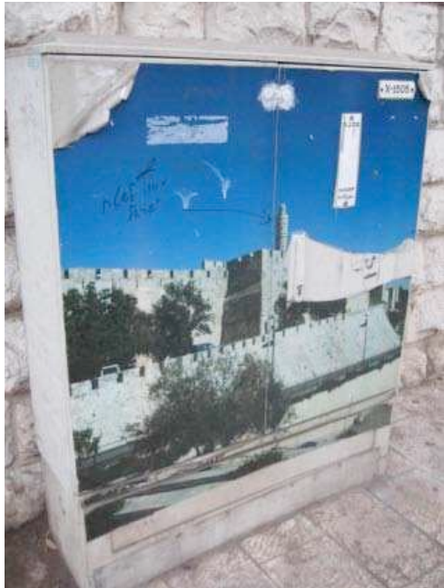
Fig. 3a: Poster on an electrical box
